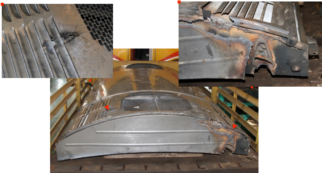
Gambar 11. Outer case system pendingan ( airconditioner ) KRL terbakar
