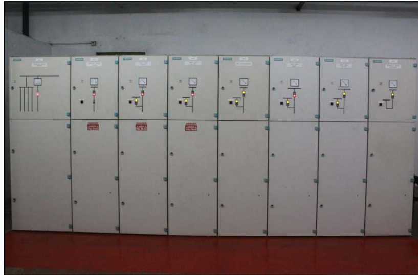
Gambar 12. High Speed Circuit Breaker
