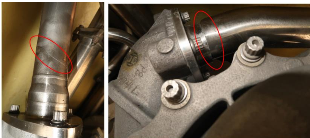
Figure 3: Fractured LP fuel tubes upstream of the Fuel Oil Heat Exchanger
