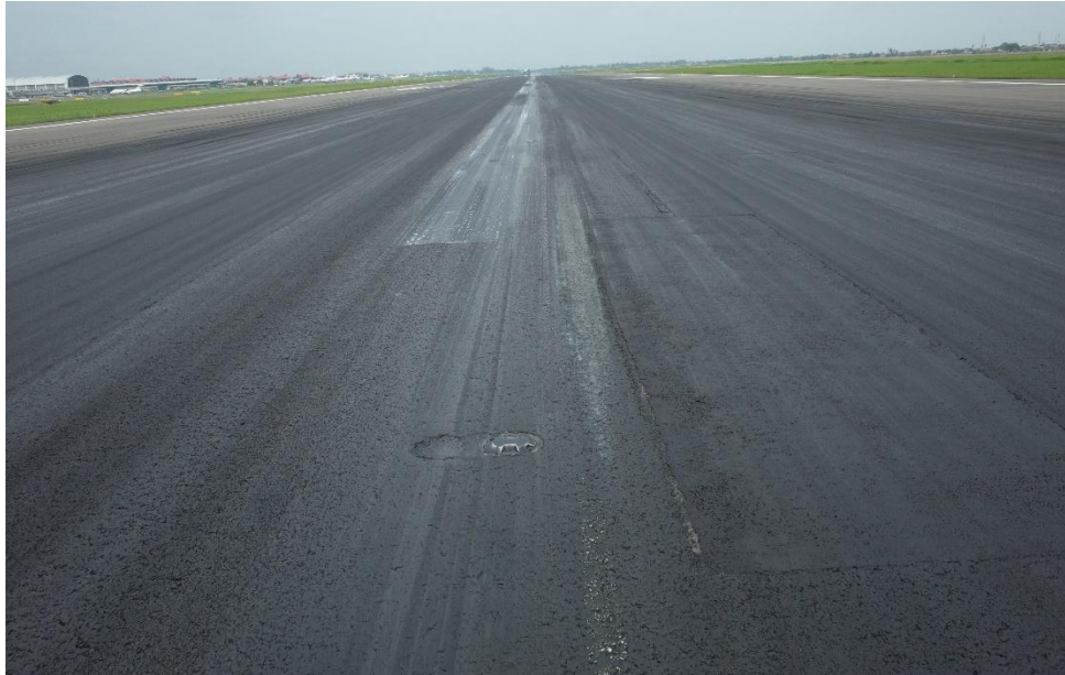
Figure 4. Thirteen meters long scratch mark on the runway
