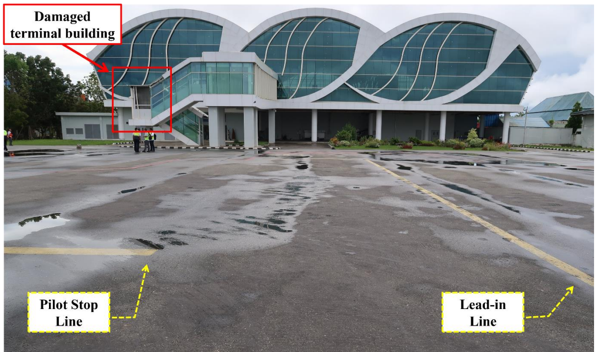
Figure 7: The damaged airport terminal building from the apron
