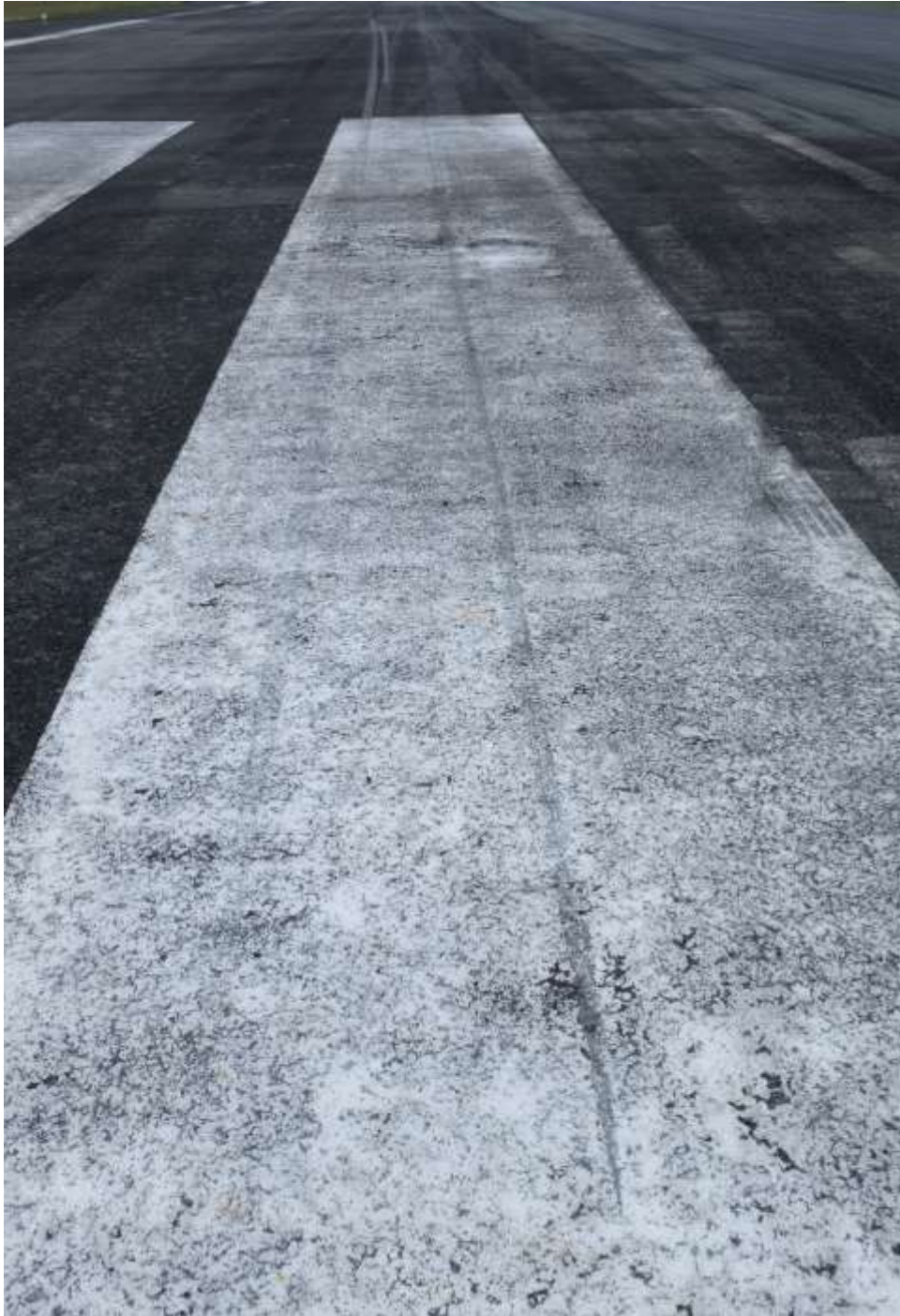
Figure 5 Fourteen meters long scratch mark on the runway
