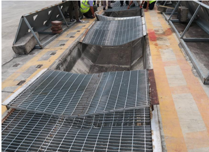
Figure 5: The damage to the ditch metal structure covers
