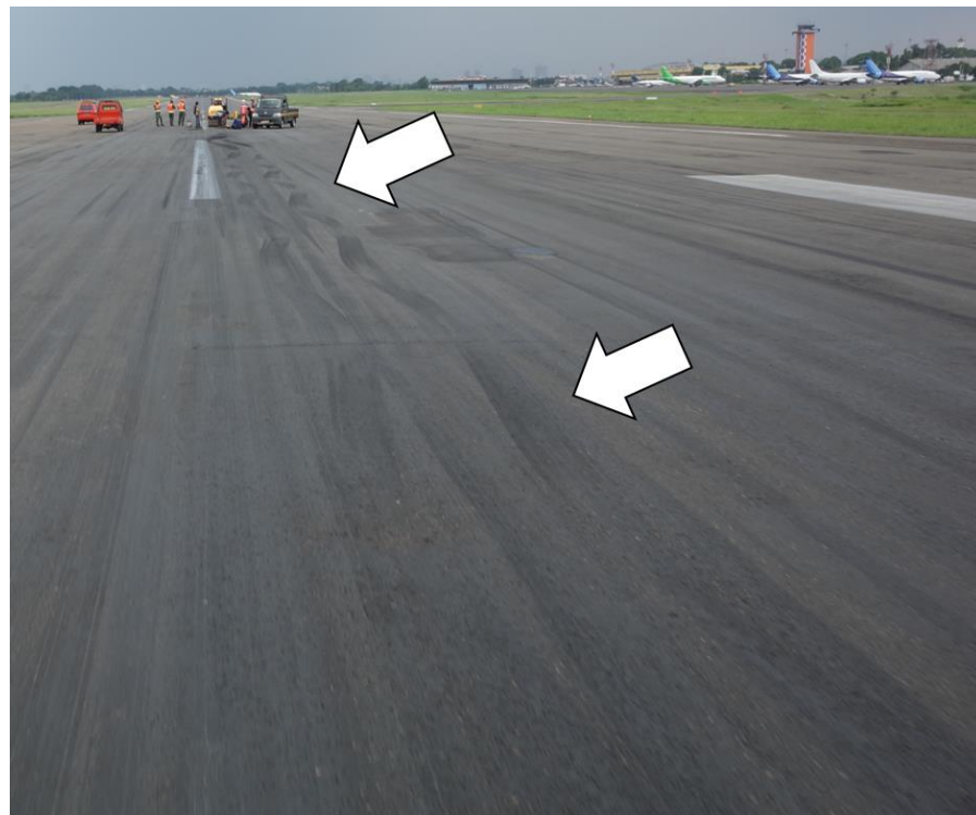
Figure 6: The zigzag tire marks of the right main wheels
