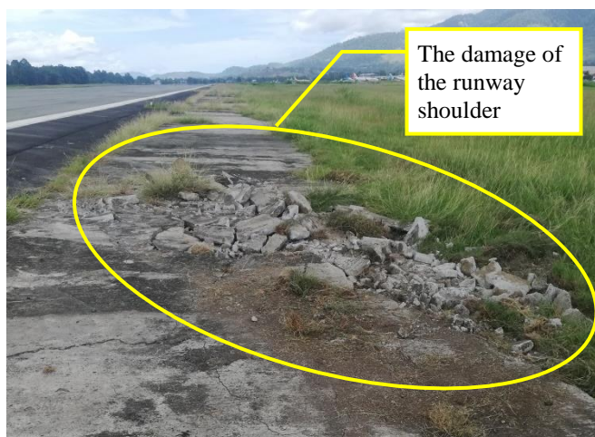
Figure 21: The damage of the runway shoulder
