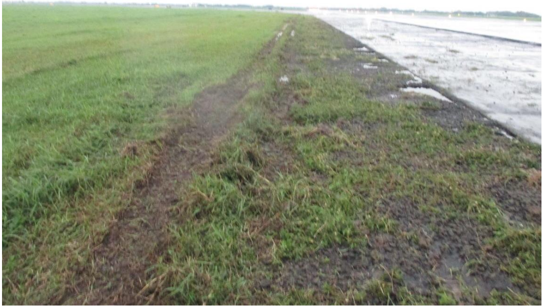
Figure 5: Wheel marks on the runway shoulder.
