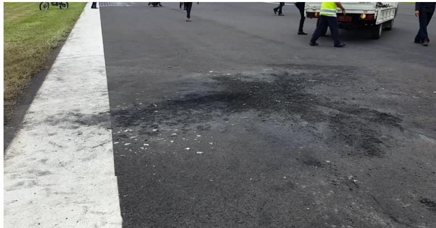
Figure 4: Heat damage on the runway
