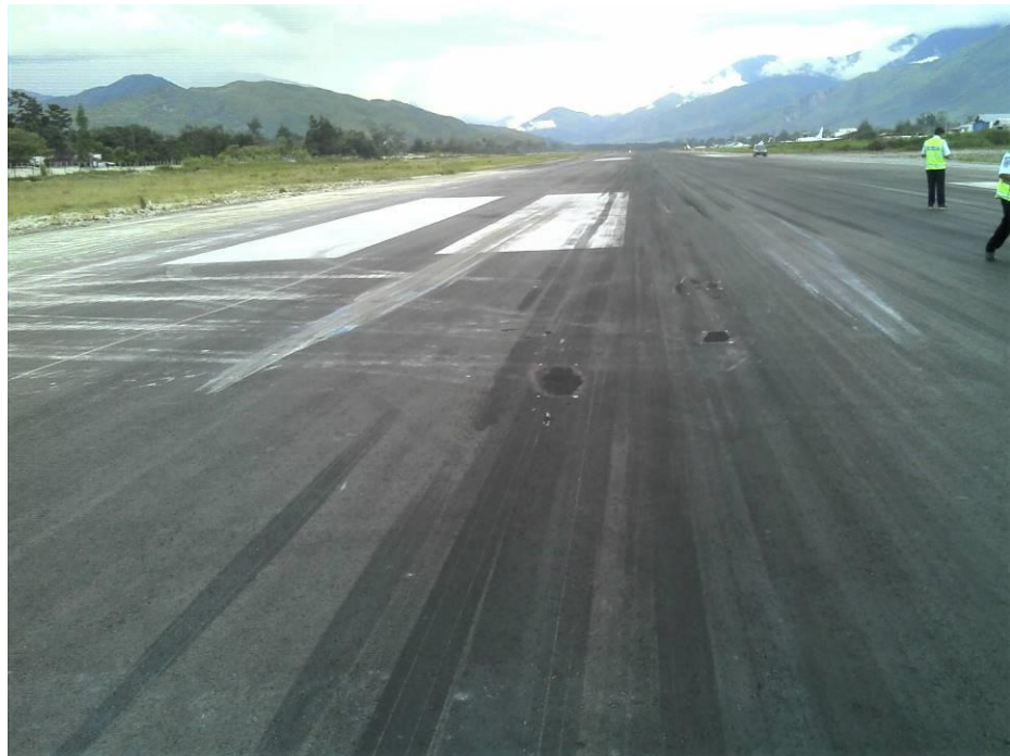
Figure 11: Marks of paint and metal scratches found on the runway
