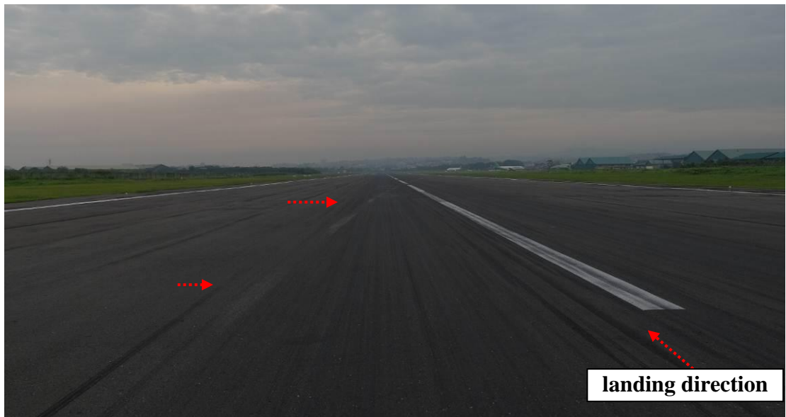
Figure 12: The white marking crossed from right to left runway centreline
