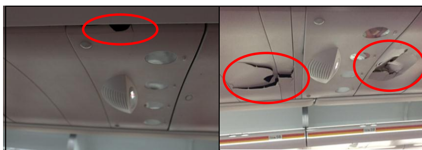
Figure 3: Several cracks on passenger service units
