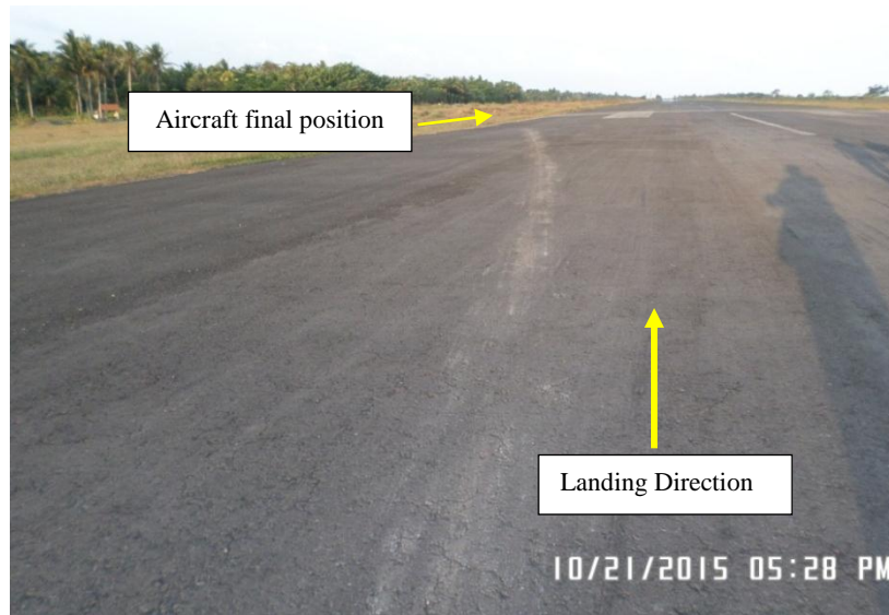
Figure 3: Metal scratch mark on the runway
