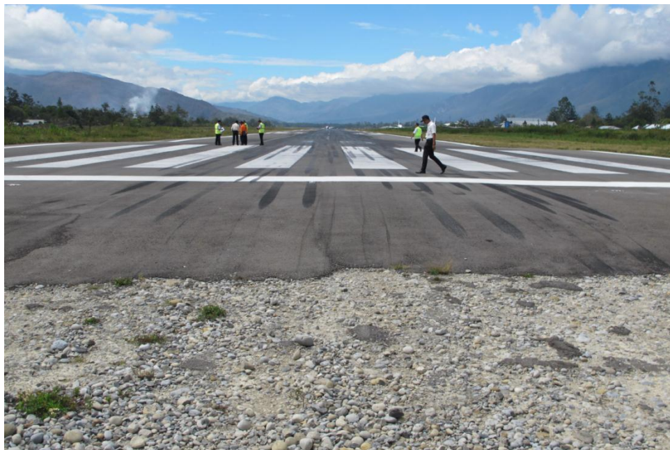
Figure 5: Touchdown marks found on the pavement before the runway 15
