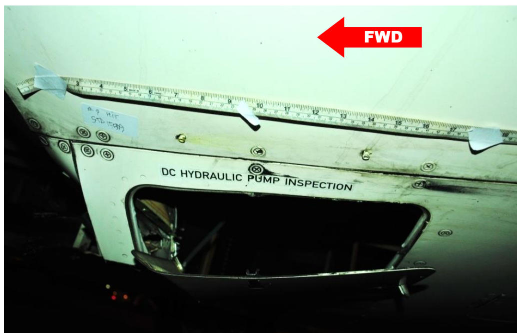
Figure 5: The hole on STA 15589
