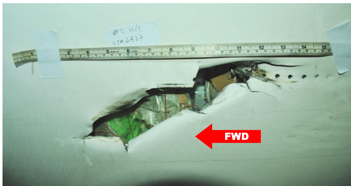
Figure 4: The hole on STA 6427
