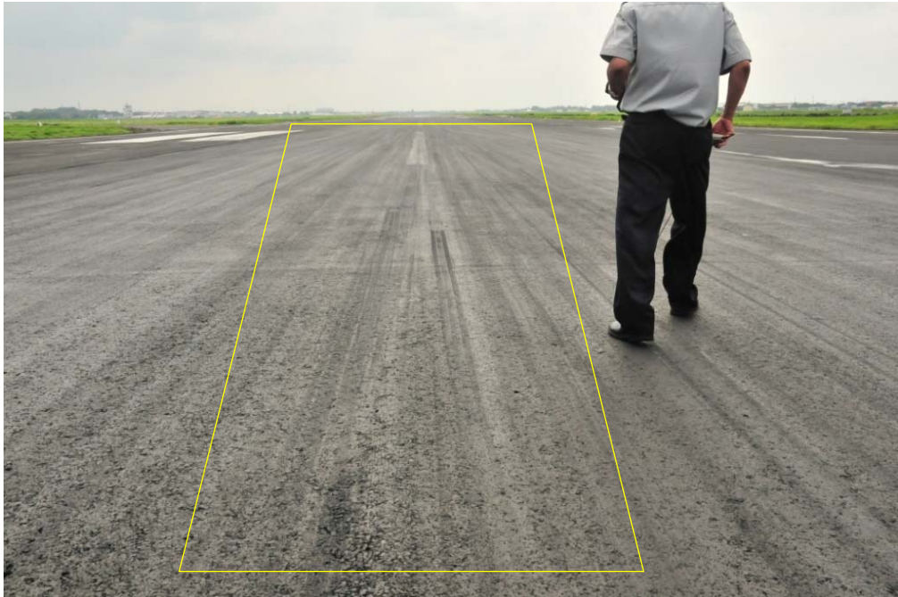
Figure 7: The centre line marking on the runway 28 covered by rubber (yellow box)
