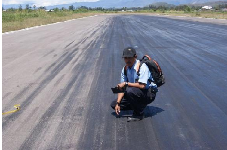
Figure 2: Surface condition on runway 33
