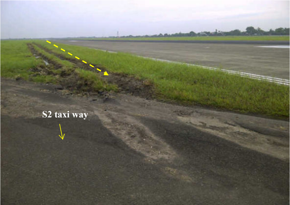
Figure 2: The right main wheel mark on runway shoulder
