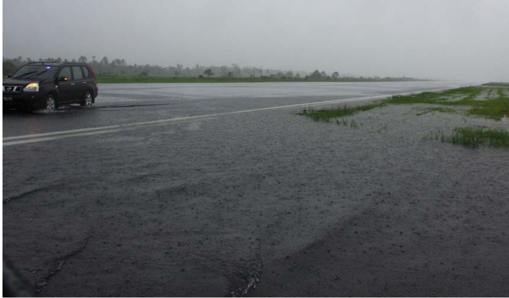
Figure 5: Standing water on intersection taxiway Charlie
