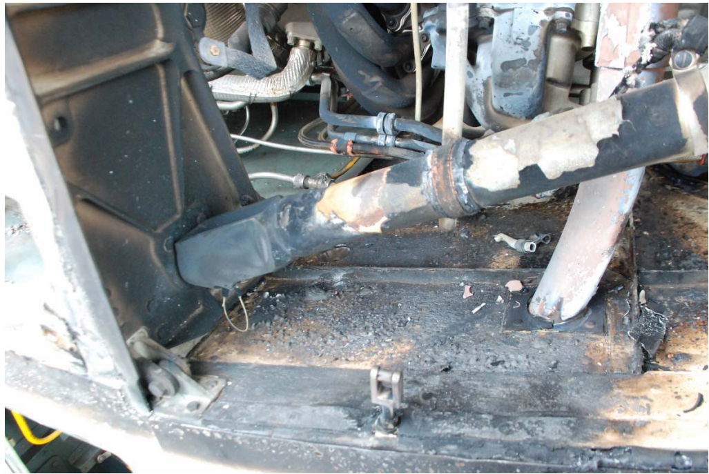
Figure 11: The most intense fire occurred on the floor just in front of the bulkhead frame
