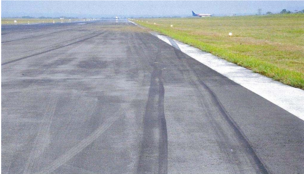
Figure7: The tire marks found on the runway
