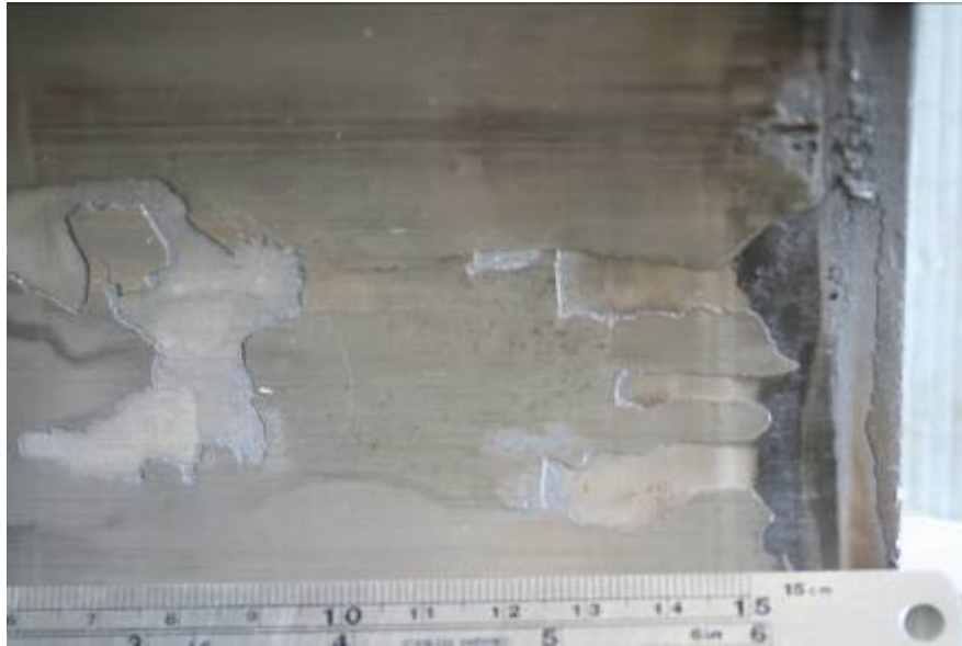
Figure 5: De-laminations started earlier from location near the TDC as indicated
