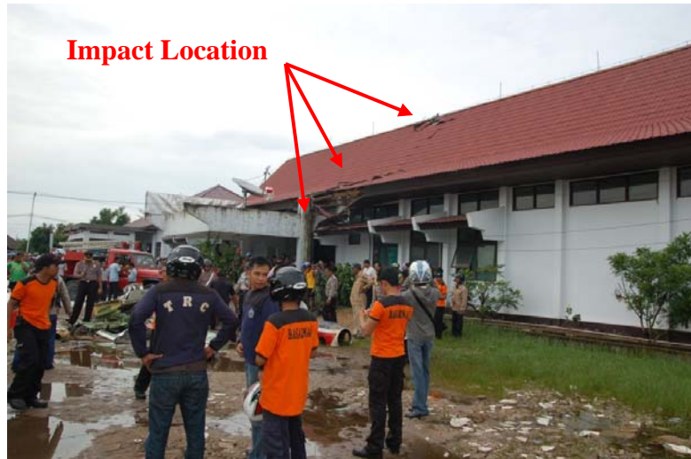
Figure 2: The hospital roof after impact
