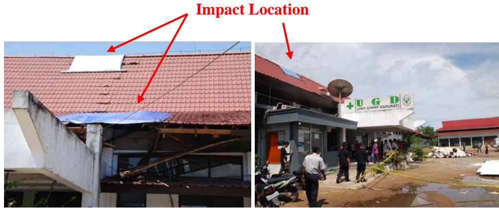
Figure 5: Initial impact on the roof of hospital
