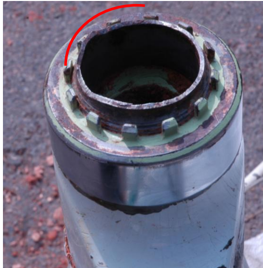
Figure 4. Corrosion found on fracture surface (red arc)
