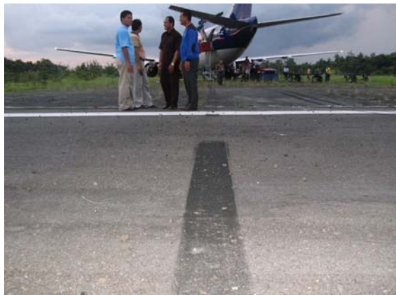
Figure 8: Tire marks at the end of the runway, and onto the stopway
