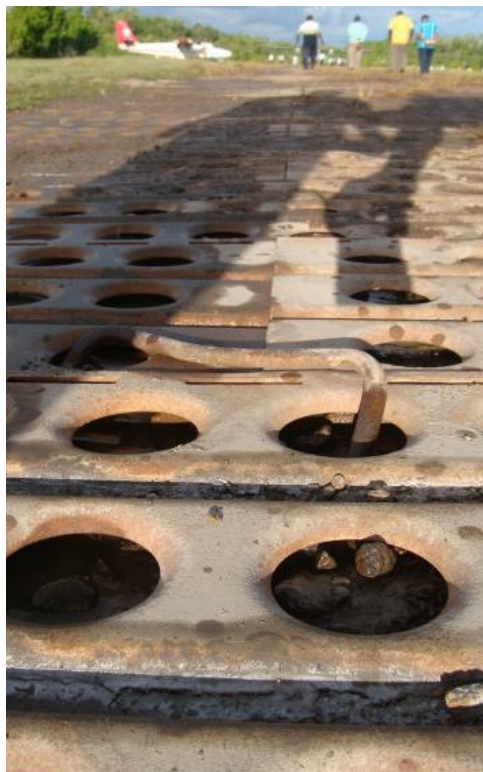
Figure 10: Marsden matting fixing pin sitting high above steel plate
