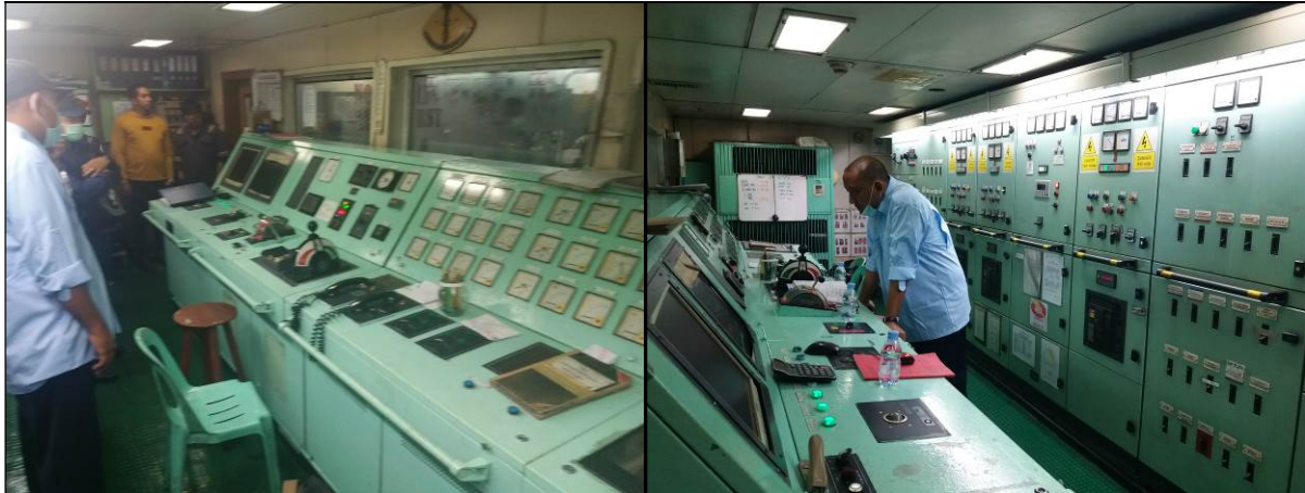
Gambar I-8: Engine Control Room Ocean River 01
