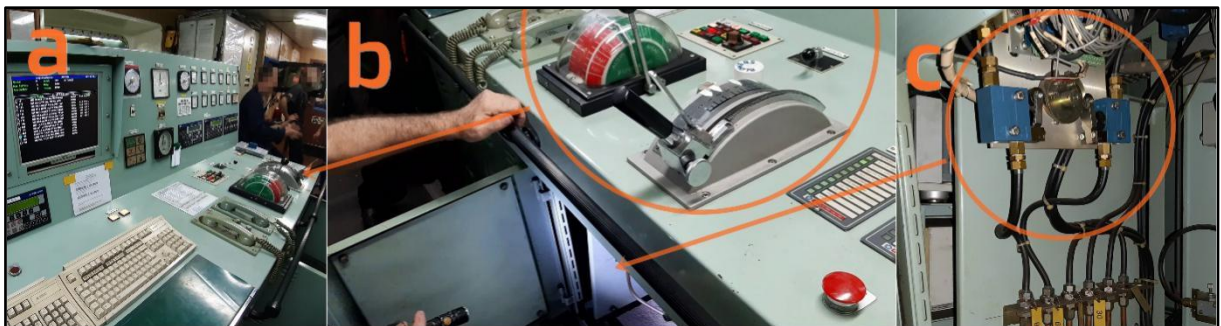
Figure II-1: The panel controls in the engine room (a); the engine control (b); the pneumatic valves
