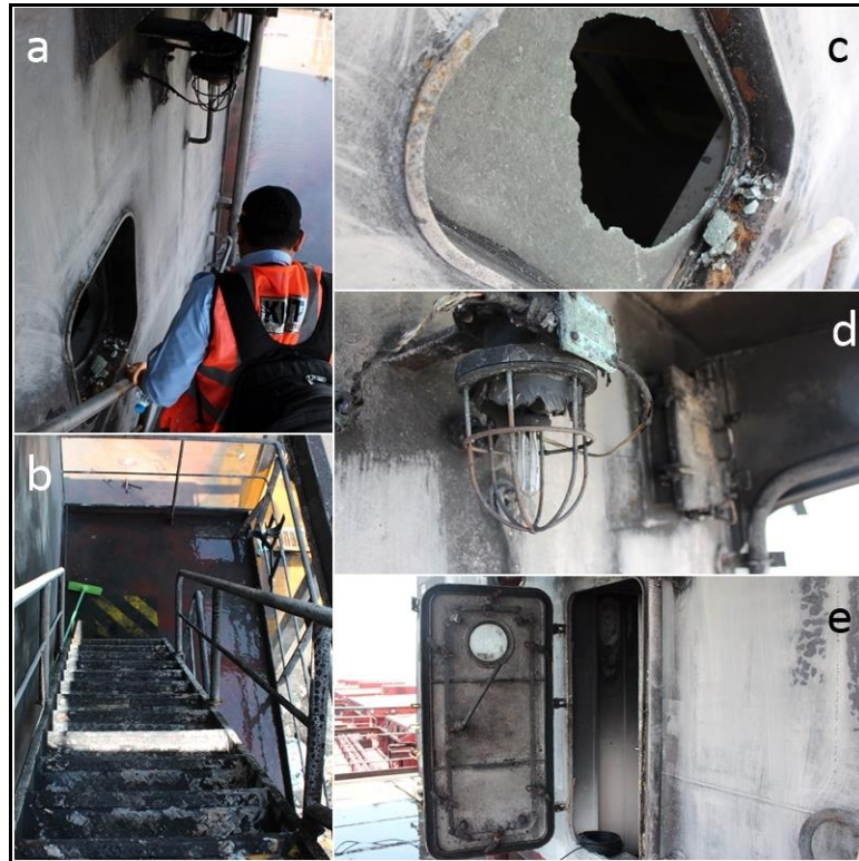
Figure I-10: a) One of the KNKT team members whilst on board; b) the sooted port side ladder; c) broken window; d) broken light; e) the sooted door
