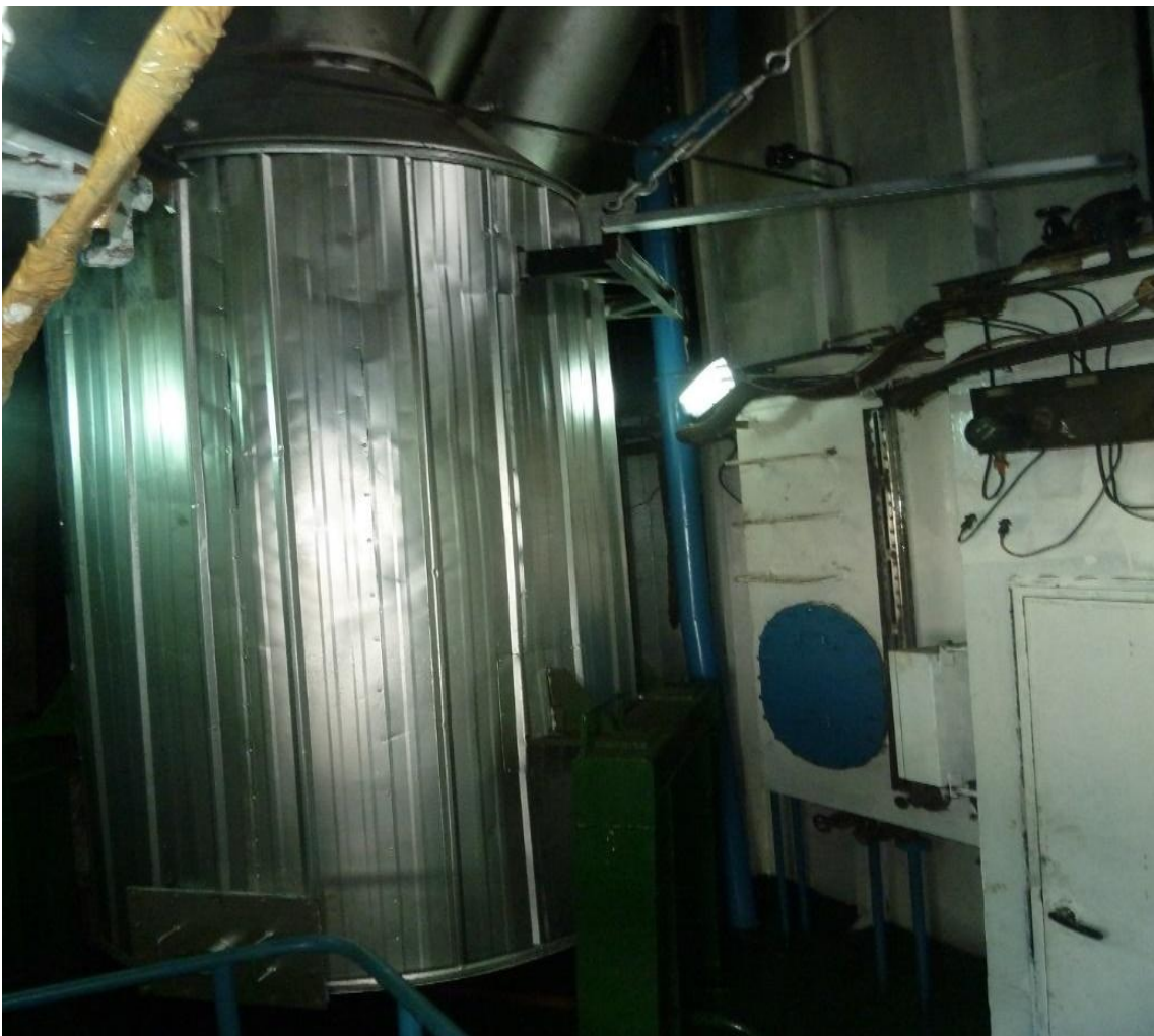
Gambar I-8: Exhaust gas thermal oil heater Pekan Fajar
