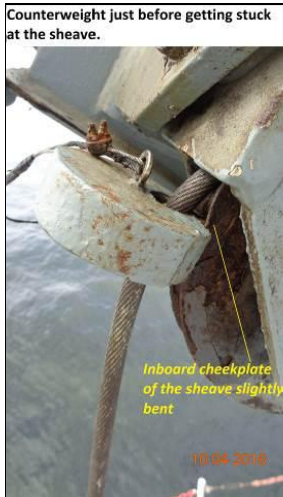
Figure II-4: Counterweight trapped against the top sheave (picture taken from company investigation report)
