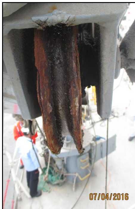
Figure I-18: Top sheave condition
