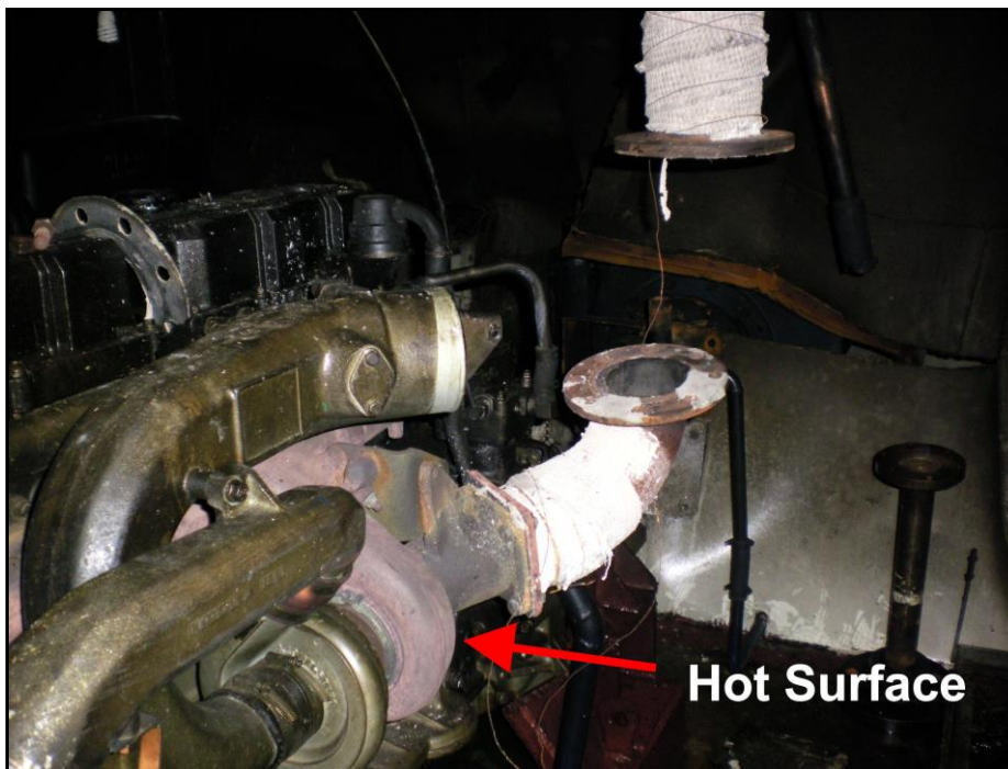
Gambar II-3: Turbocharger dan manifold gas buang Mesin Pompa Muatan no. 3
