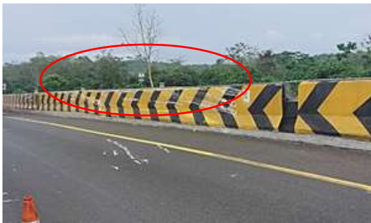
Gambar 28. Scratch marks di median jalan KM.92+200B
