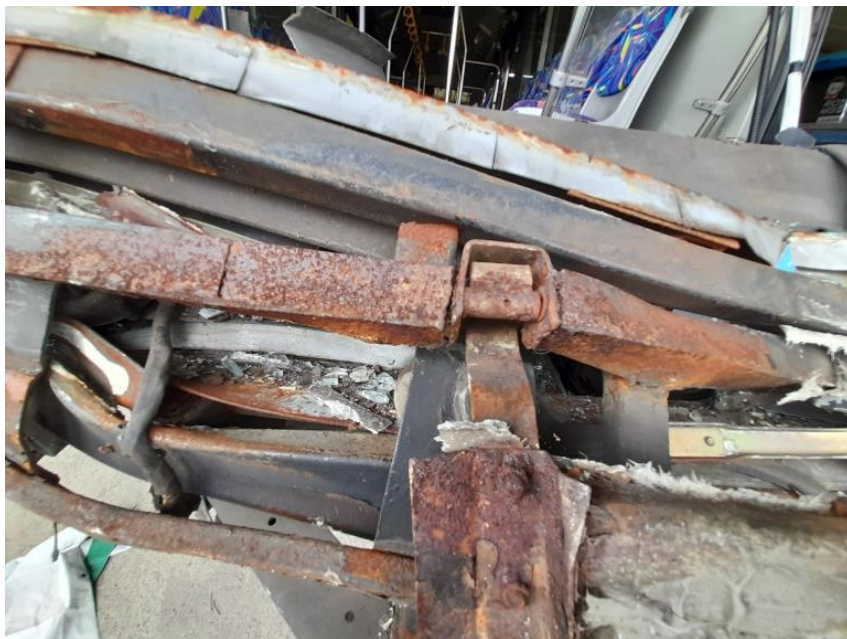
Gambar 5: Kondisi Kerangka Superstructure Bus 1
