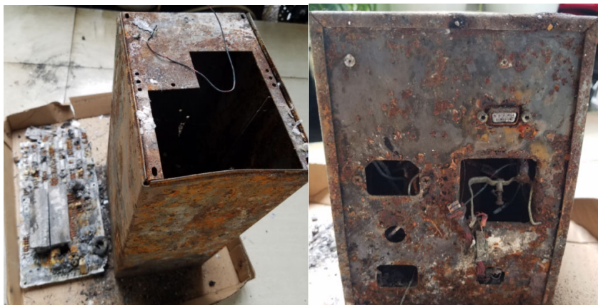
Gambar 8. Power Inverter pasca mobil bus terbakar
