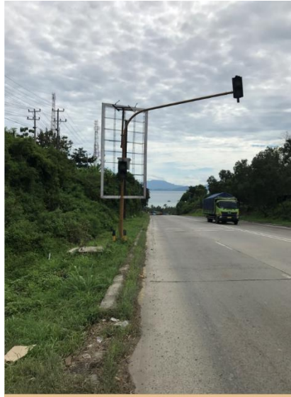
Gambar 17. Lampu Peringatan ( Warning Light )
